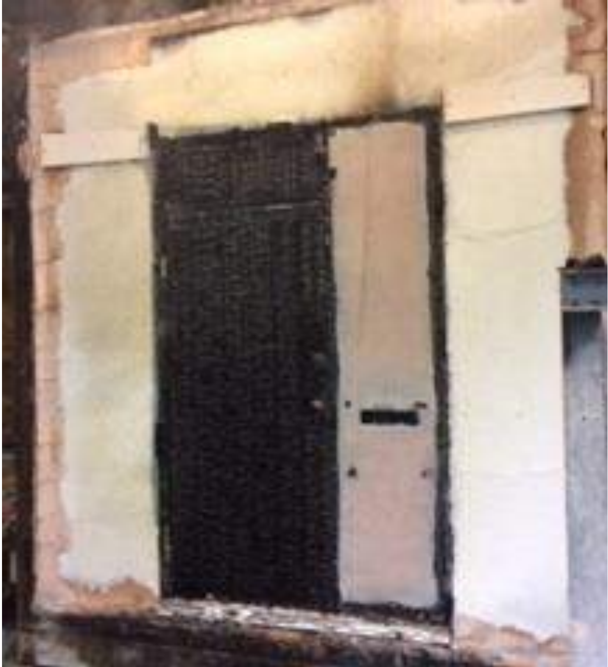
Exposed face – post test
